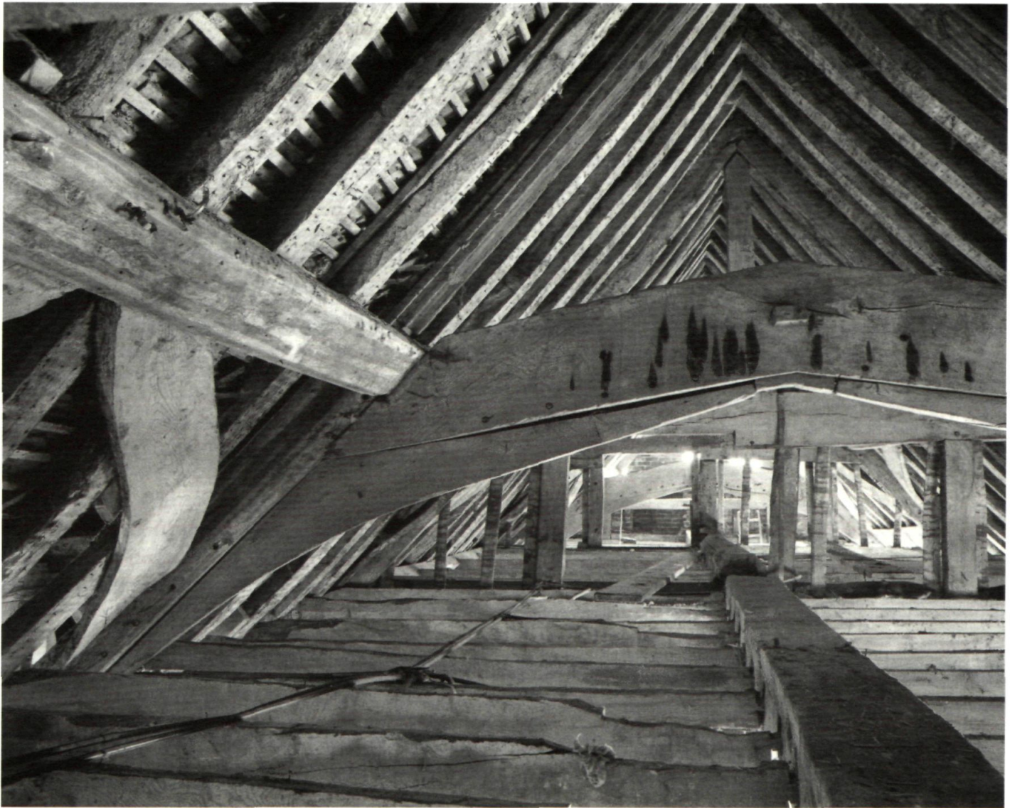
Plate 3. Abbots Barton Farmhouse, showing the main trusses with queen struts, and the intermediate trusses with arch-braced collars. The secondary, attic floor has recently been removed. (Photo – John Crook)
