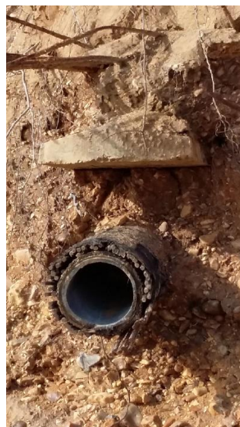
Remains of a pipeline in the cliff
