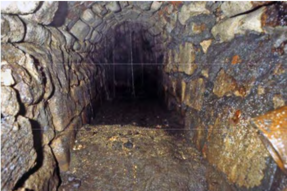
Fig. 16 The Lockburn under south end of No. 9 The Close showing probable eleventh-century side walls and vault. Photo : J Crook
