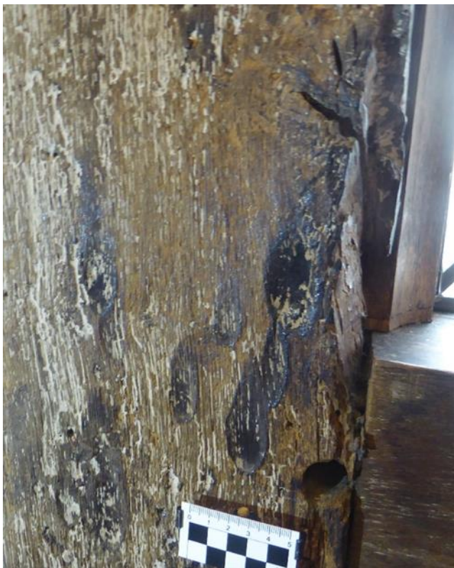
Fig 21. Timber upright, east side of top of stairs. Taper burn marks
