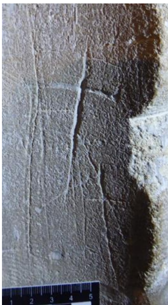
Fig 4. North doorway, west jamb. Crosses
