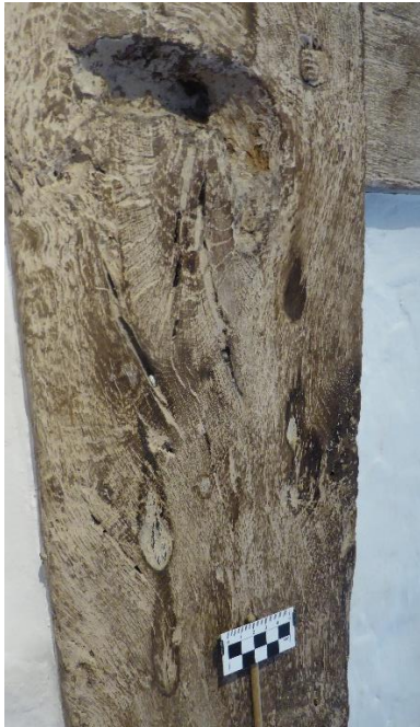
Fig 20. Timber upright, west side of top of stairs. Taper burn marks
