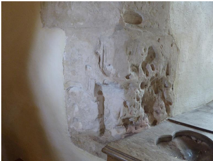
Fig 6. South window 1, east jamb. Weathered stone
