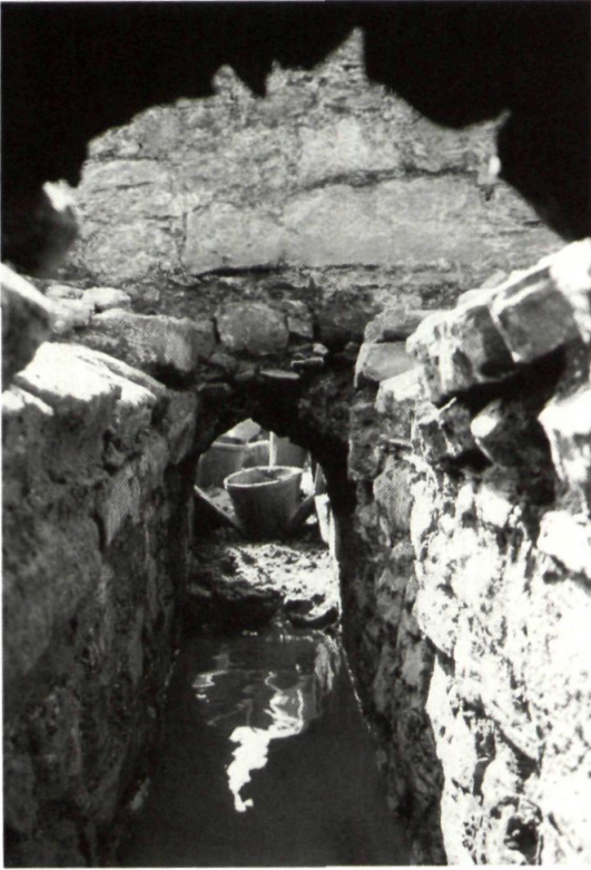
Fig 11. View west along the channel of the Annexe, from inside the arched drain. The capping slabs have been removed.
