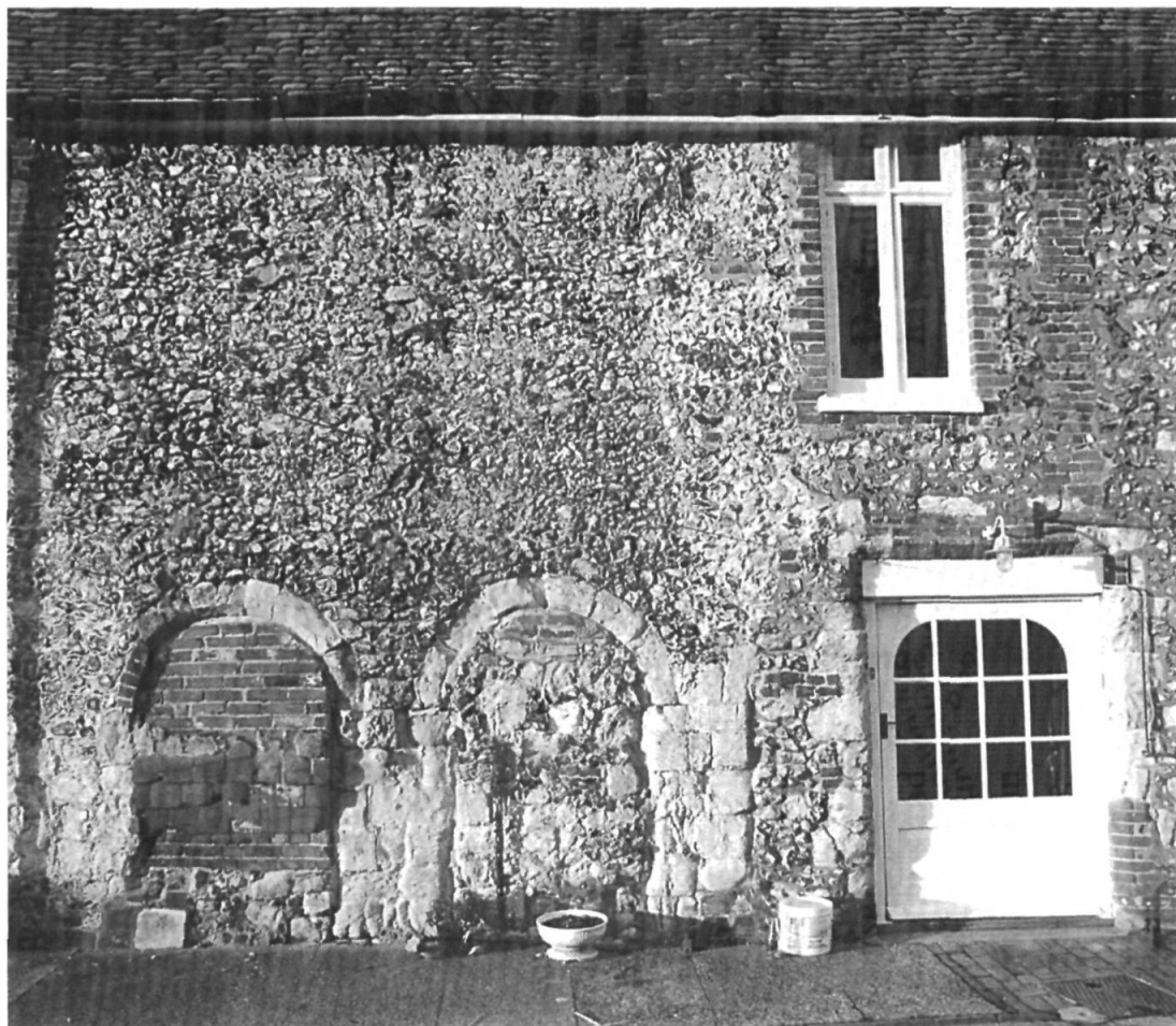
Fig. 3 Two round-headed doorways with a jamb and springing of an arch for a third doorway (right) in the south elevation of the larger, western block. (Winchester Museums Service, PWCM 21509: © John Crook).
