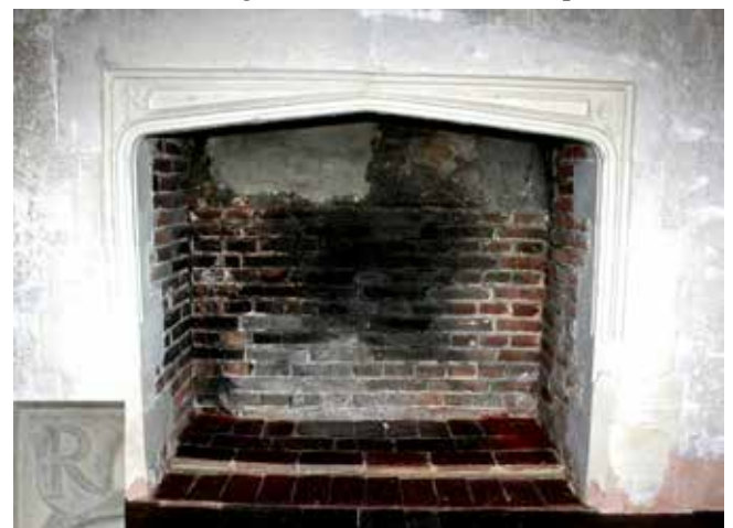
Fig. 2. A first-floor fireplace with the initials ‘R’ (see inset) and ‘O’ in the spandrels, signifying Sir Robert Oxenbridge.
