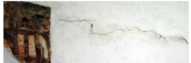
Fig. 4. Cracks in the plaster at the edge of the wall paintings.
