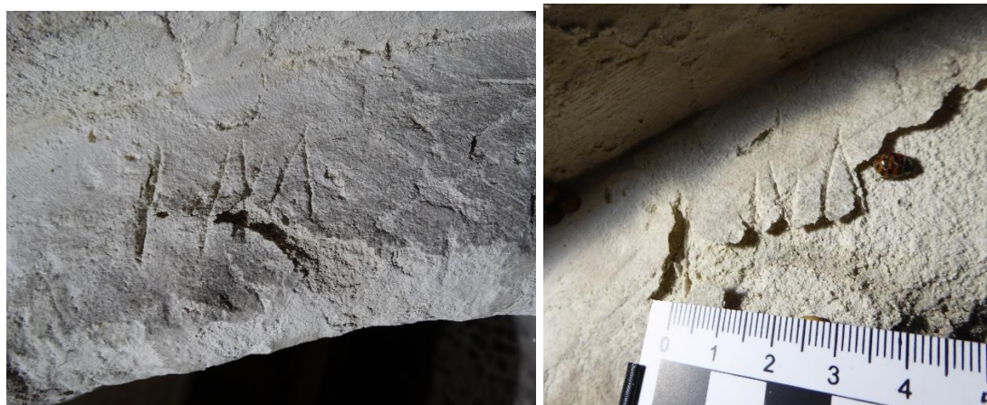
Figs 1 and 2. Clock chamber doorway arch. Graffiti initials IM in 2016 and 2026 showing significant loss
