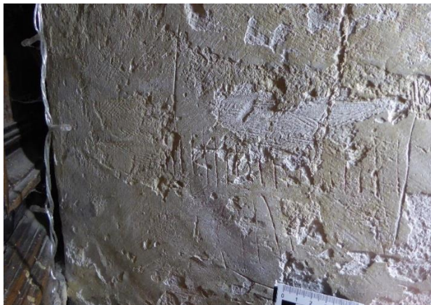
Fig 47. North of chancel arch. Marks on plaster next to pulpit steps
