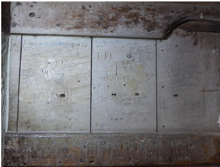
Fig 40. Ringing chamber. Main door. Top panels (panels 5-8) with graffiti
